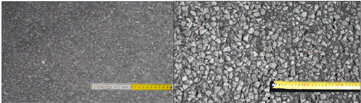
Figure 3. Picture of the SMA11 road surface (left) and the SMA16 road surface (right)
